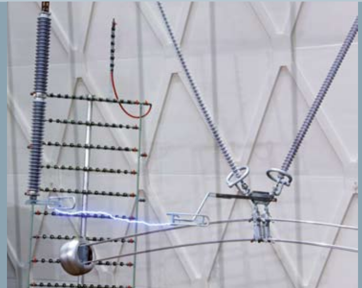
Type test on a 400-kV EGLA line surge arrester
